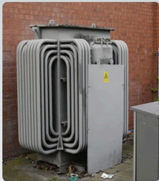
local substation live data / power support
