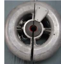
Power Donut fitted to 132kV conductor – measures conductor current and temperature
